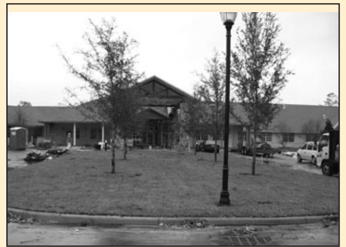
LUTHERAN HAVEN CLOSER TO MOVING IN — Paint, wall-coverings, carpet and landscape are the finishing touches under way as residents of Lutheran Haven in Oviedo, FL, gets closer to moving into their new nursing home and assisted living residence. Projected move-in date is mid-November. Dedication is Sunday, January 22, 2006, at 3 PM. □
